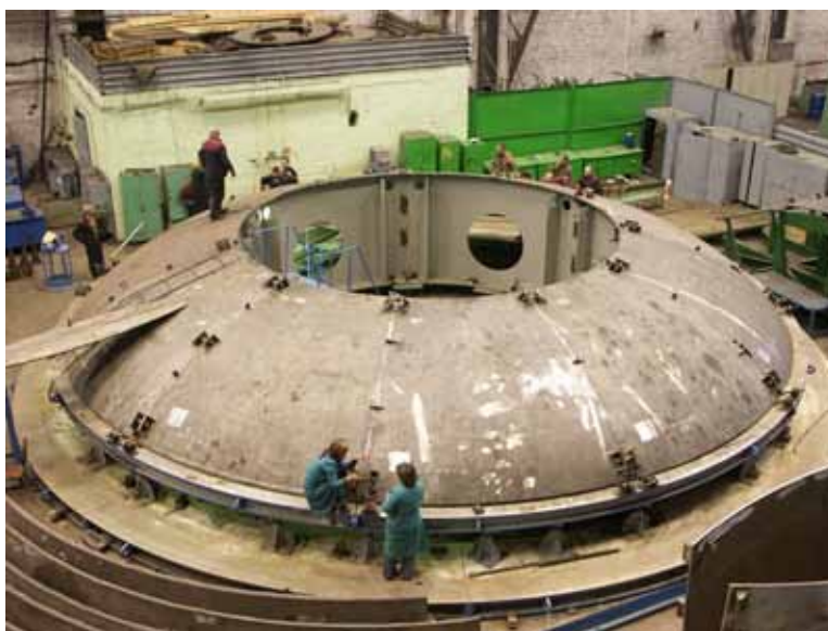
Reactor vessel for the BN-800 fast neutron reactor, under construction in Russia. When large-scale deployment of such plutonium-breeding reactors will be needed depends on how much uranium ultimately proves to be economically recoverable and how fast nuclear energy grows in the future. Source: JSC Machine-Building Plant ZiO-Podolsk.
