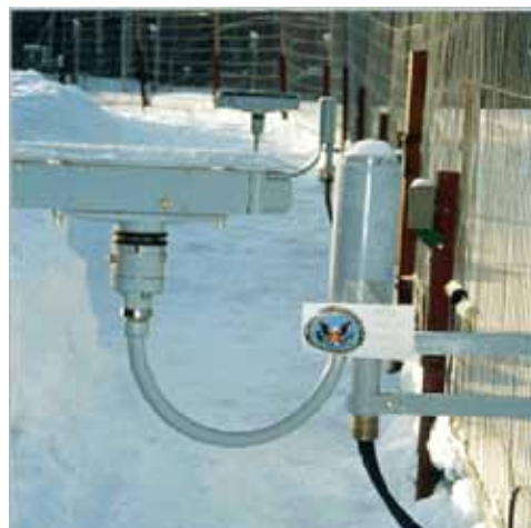
Upgraded fencing and intrusion detectors at a nuclear site in Russia. U.S.-Russian cooperation has led to major improvements in security for nuclear weapons and materials, greatly reducing risks to the security of Russia, the United States, and the world.
