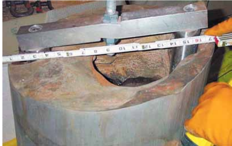
A football-sized hole in the pressure vessel head of the U.S. Davis-Besse nuclear plant almost led to a large loss-of-coolant accident. Such incidents make clear that even the countries with the most nuclear experience need to continuously struggle to strengthen safety culture. To keep accident risks from rising as nuclear power grows around the world will require achieving ever-higher standards of safety, requiring new technical and institutional approaches. Source: FirstEnergy
