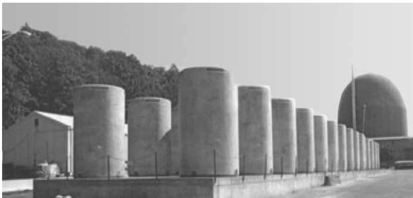
Figure 14.15 | Dry cask storage of older spent fuel at a US nuclear power plant. Each year, a 1000-MW e light-water reactor discharges spent fuel that originally contained about 20 tonne of uranium. Each cask typically holds about half that amount and costs US 2005 $1–2 million. Reprocessing spent fuel costs about ten times as much. Source: Connecticut Yankee, 2008.
