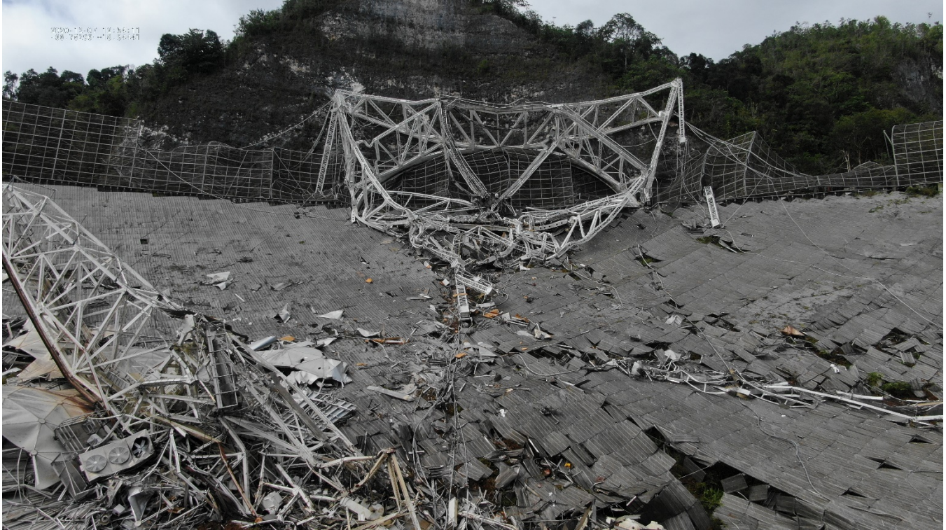
Figure 1. Platform structure hanging on the rim wall following collapse. The committee recommended salvaging samples of main components, such as platform corners, azimuth and zenith track portions, rotary joint and beams sections.
